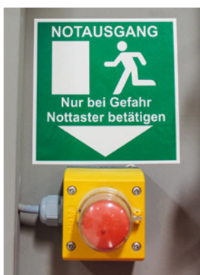
Emergency open switch
