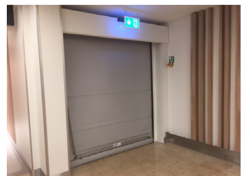
Emergency exit door without viewing window
