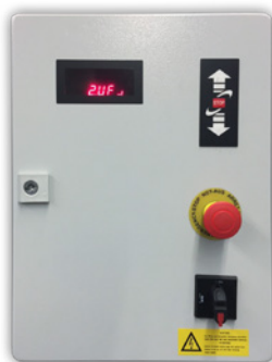
Control for emergency exit doors
