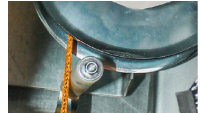
Monitoring sensor for counterweight
